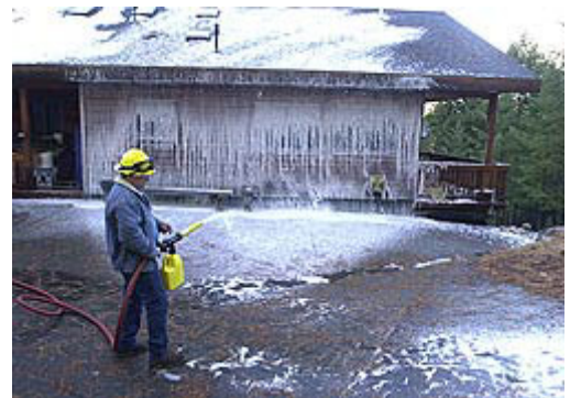
David Evraiff demonstrates his Home Firefighting System on his Pollock Pines home. Evraiff is a self-taught electrical and mechanical engineer who began marketing the system in 1999 after developing it for his own home in El Dorado County.
